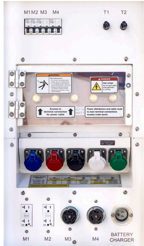
Convenience receptacles, weathertight camlock connections
